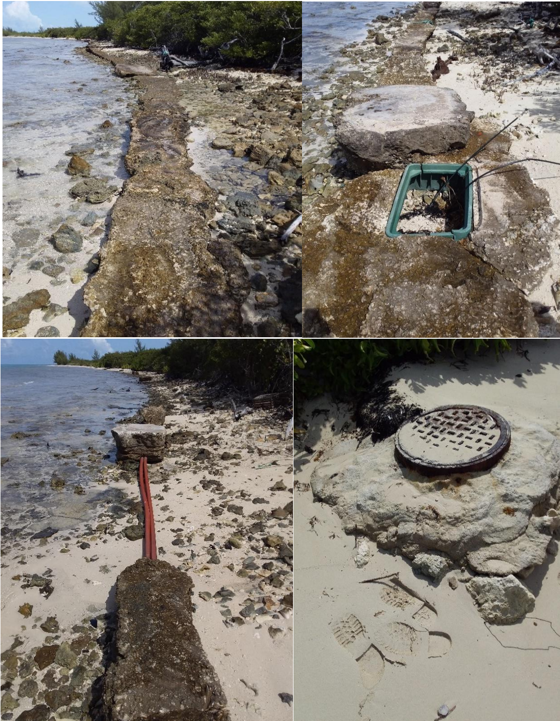
Figure 7.163. Exposed ICT cable infrastructure along western shoreline of Leeward Harbour (2018).
