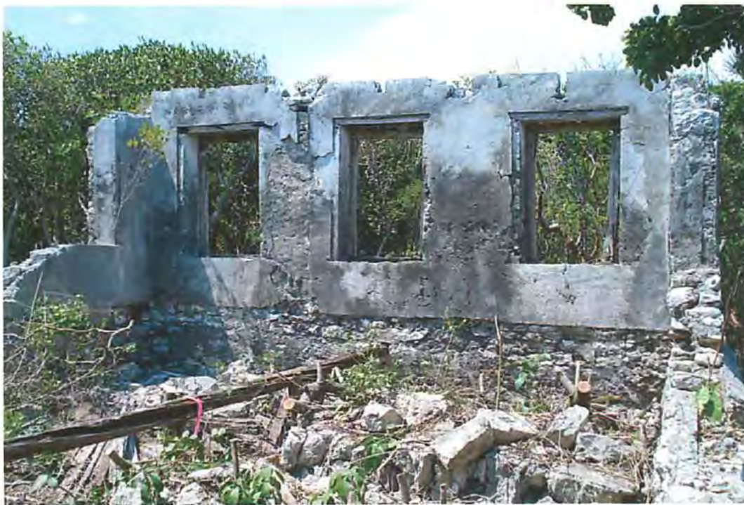
Figure 54, Barque Bay Structure 4, interior view showing beam for joists supported by cedar posts and slots at top of north wall for rafters, toward northwest
