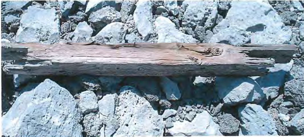
Figure 24, Lantern Head Structure 1, Head of window frame found loose in ruin
